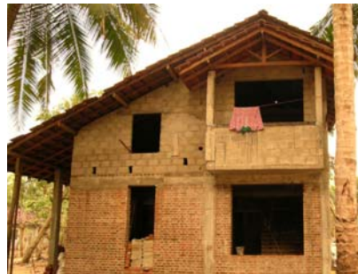
Fig. 1 - Typical damage to masonry dwelling (Courtesy of EEFIT)
